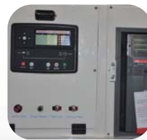
Control Panel & MCB
